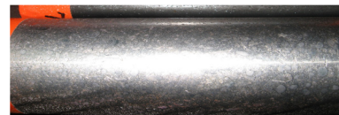
Figure 10: No corrosion products on nCoP-coated steel bars following exposure to 30 days magnesium chloride salt spray testing.
