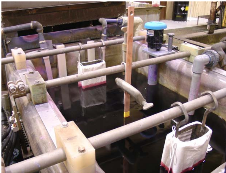
Figure 9: 250 gallon nCoP dem/val plating tank at FRC-SE
